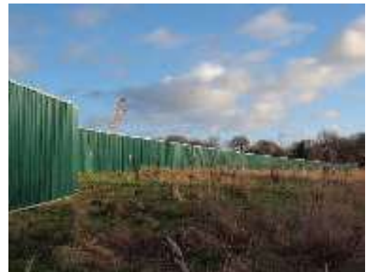
Figure 15 Sound barrier is used as part of the noise dampening control to minimise disturbance to neighbouring communities.
